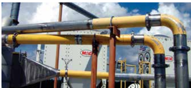
Solvay paints Kennametal components yellow to distinguish them from unprotected piping.
