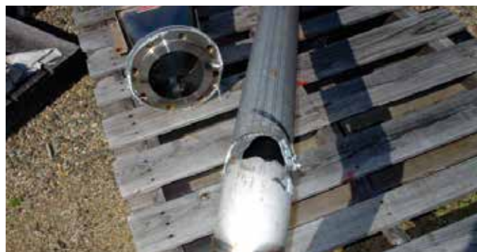
Elbow and pipeline blowouts were common before Solvay installed Kennametal conveyance components.
